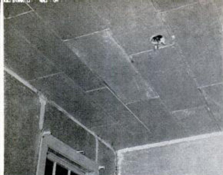
Original ceiling is completely covered with gypsum lath and ready for new plaster. Only a 1/2-in.-thick layer of plaster is required to cover the lath base
